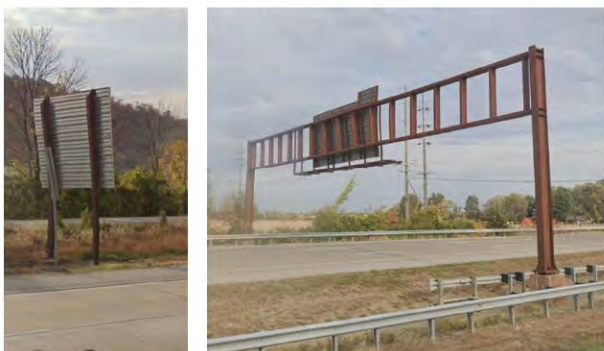
Left: Sign supports along I-255 have the same earth tone color as the bridge girders.
